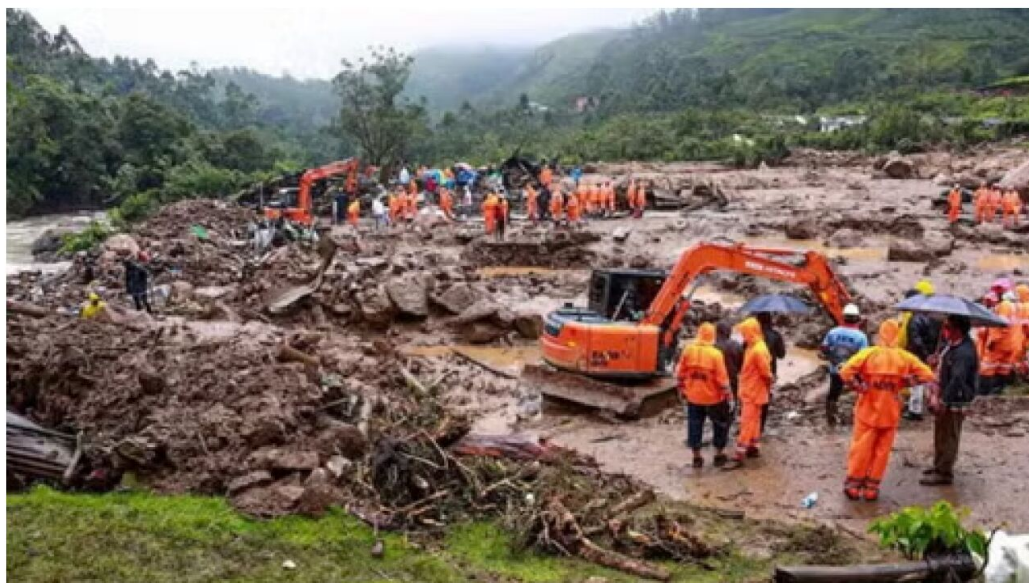
Human activities – such as construction in eco-sensitive regions – are making many hilly areas more susceptible to landslides (AP)
